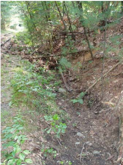
Figure 17: Visible Erosion Adjacent to Railbed
